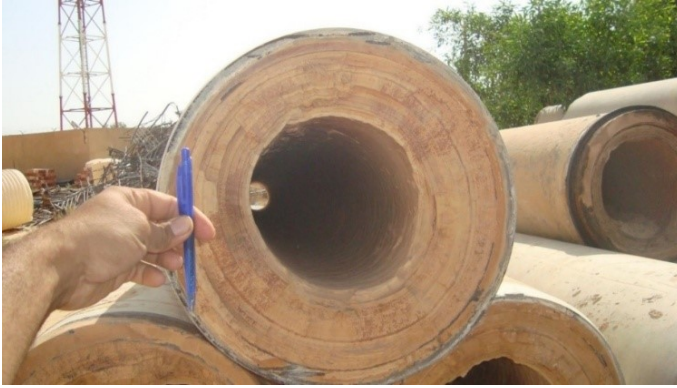
Figure 13: The condition of the drinking water supply network pipes in the town of Touggourt after 7 to 8 years of service (Remini and Amitouche, 2023a)
