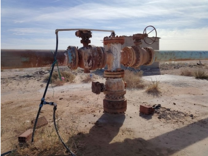
Figure 15: El Oued, Albian borehole over 1800 m deep (Photo. Remini, 2024).
