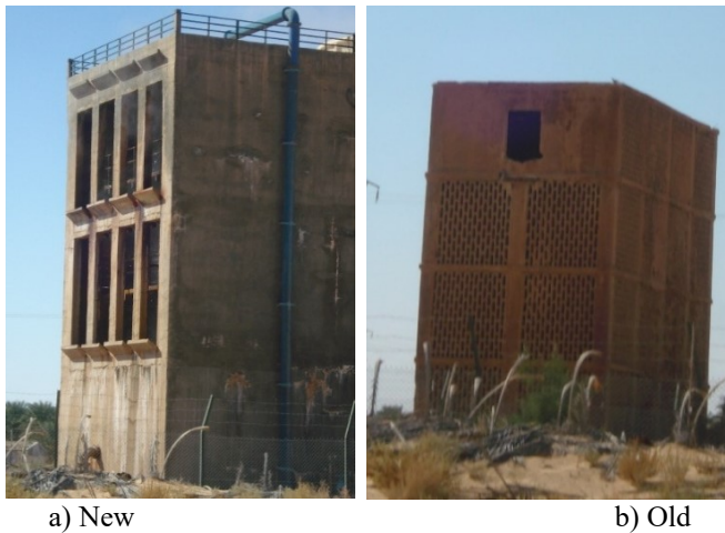
Figure 12: Cooling tower for the brackish waters of the Continental Intercalaire in the Oued Righ valley (Photo. Remini, 2010)
