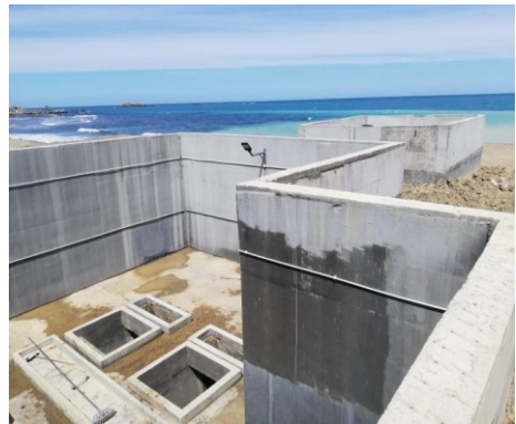
d) Pumping basin
