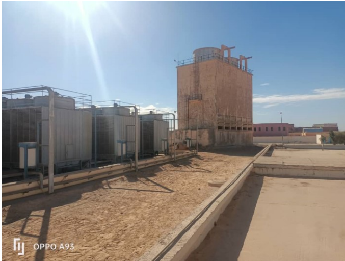
Figure 16: A cooling tower for Albian aquifer water before it reaches the reverse osmosis process at the El Oued demineralization plant (Photo. Remini, 2024)
