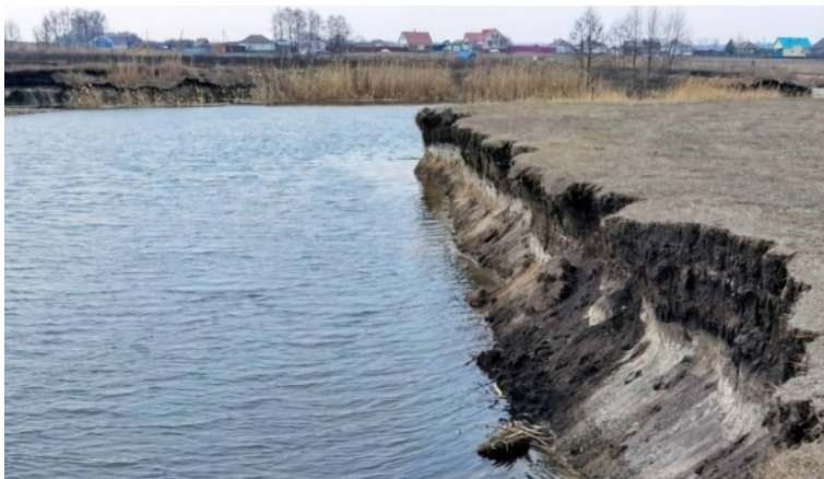
Photo 1: Damage to slopes caused by water flow on coastal slopes
